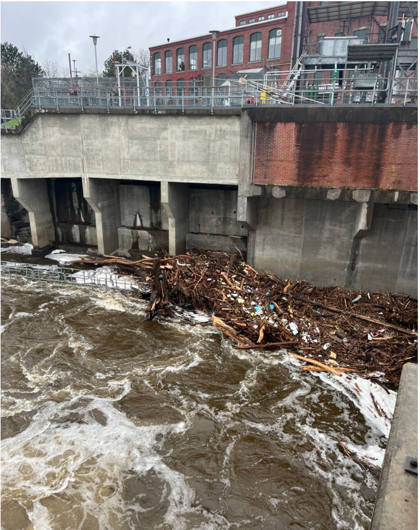
The Brunswick Project vertical slot upstream fish passage pictured above.
